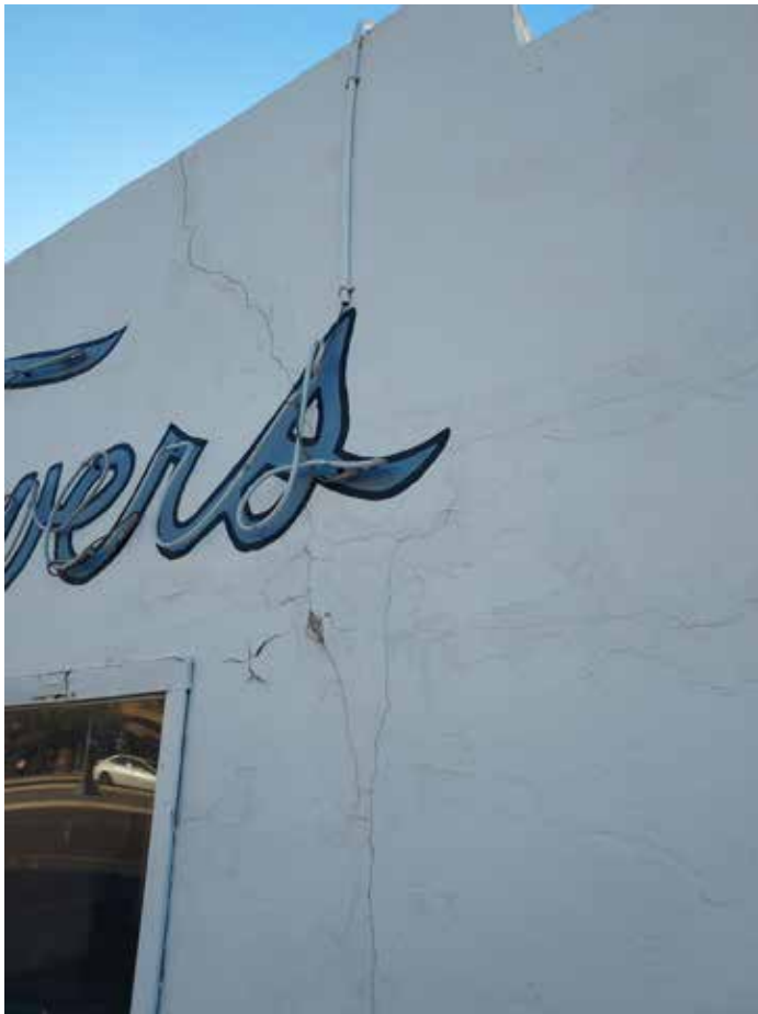
Crack at north wall
