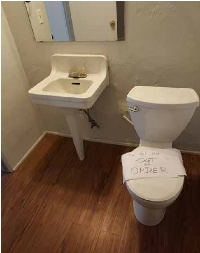
Powder room fixture
