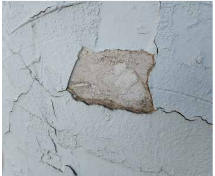
Cracking paint buildup close-up
