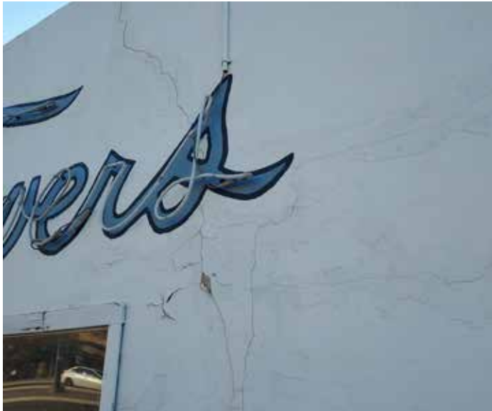
Crack at north wall
