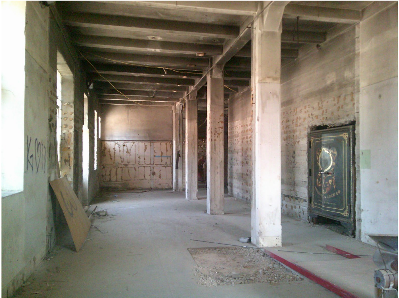
Photograph 5. Detail of ground floor room on south half of mill building showing recessed safe, view facing north (AZ_MaricopaCounty_HaydenFlourMill_005)
