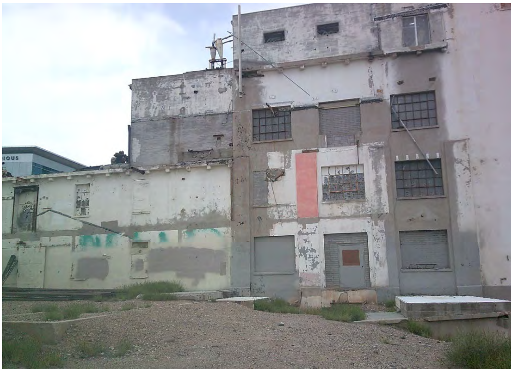
Photograph 12a. Resource No. 2, concrete footers of wooden addition and cribbed wood tower against mill building foundation, view facing southeast (AZ_MaricopaCounty_HaydenFlourMill_012a)
