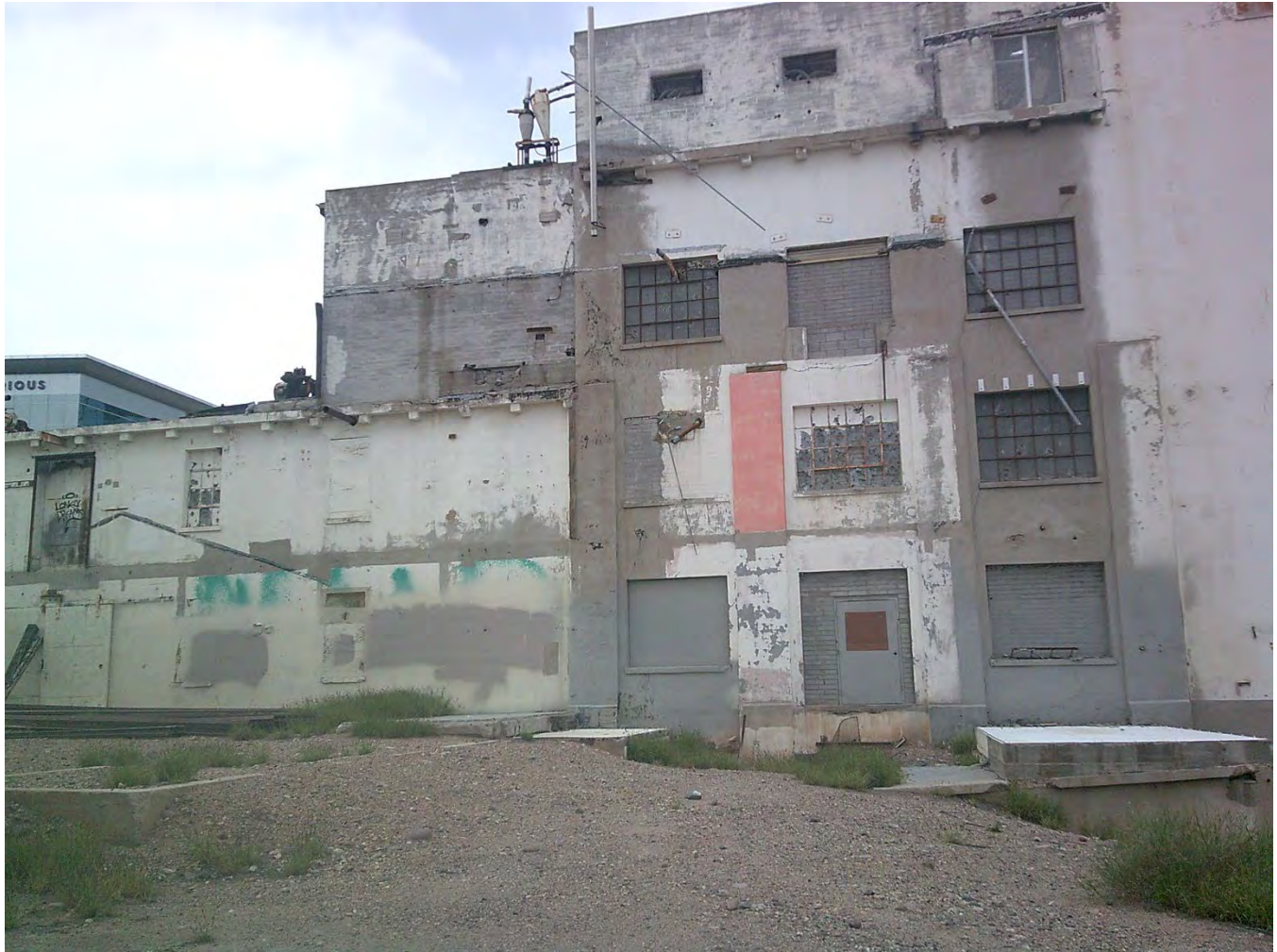
Photograph 12a. Resource No. 2, concrete footers of wooden addition and cribbed wood tower against mill building foundation, view facing southeast (AZ_MaricopaCounty_HaydenFlourMill_12a)
