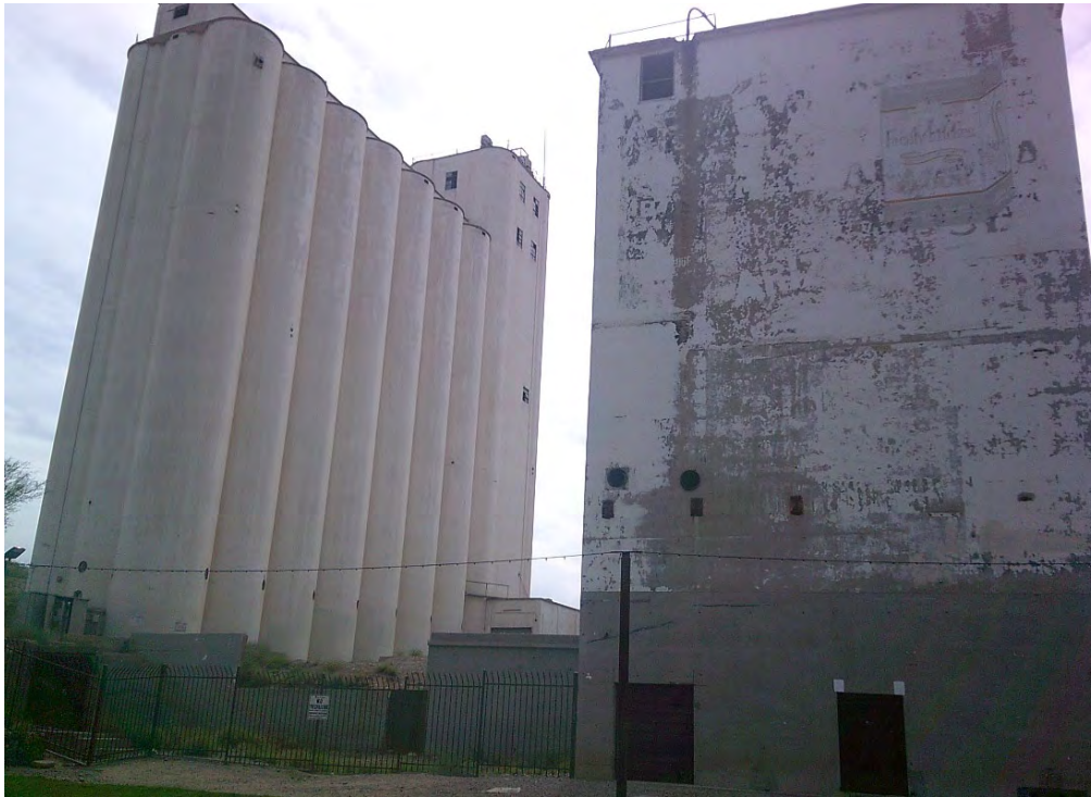
Photograph 10c. Overview of silos and grain elevators north elevation, view facing southeast (AZ_MaricopaCounty_HaydenFlourMill_010c)
