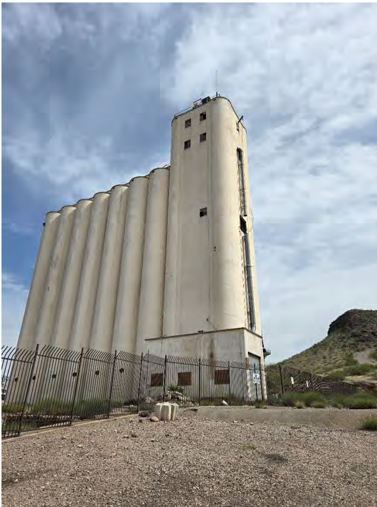
Hayden Flour Mill Silos, west elevation, view facing northwest (WestLand Engineering & Environmental Services, March 14, 2024)
