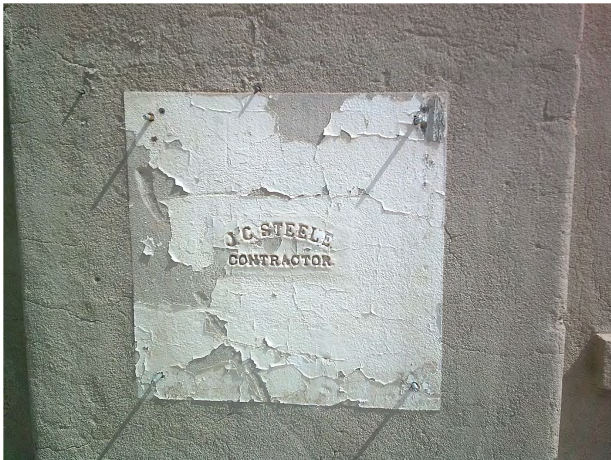
Photograph 15. Detail of contractor's stamp on the west elevation, view facing east (AZ_MaricopaCounty_HaydenFlourMill_015)
