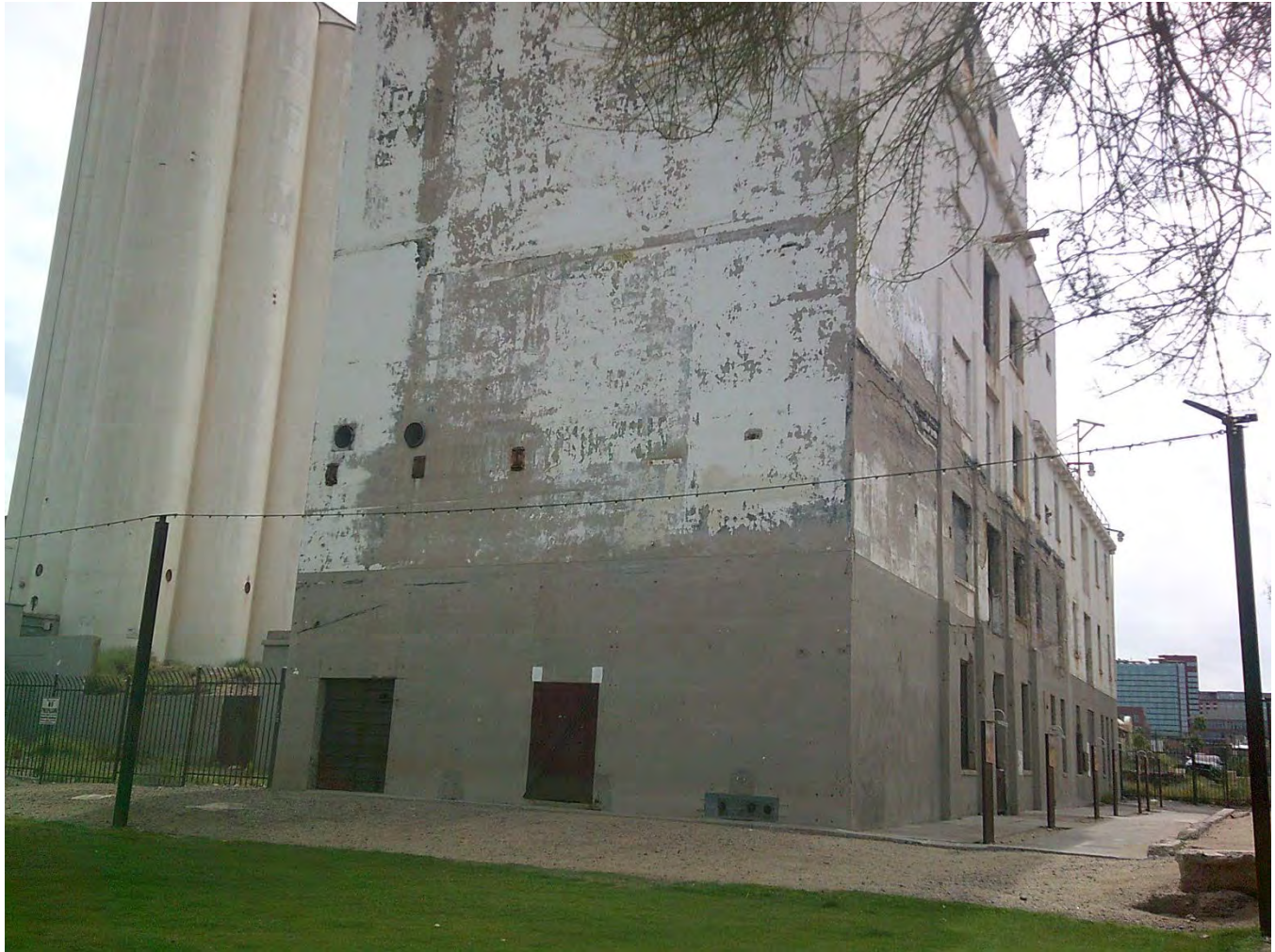
Photograph 2c. Overview of the north elevation of mill building, view facing southeast (AZ_MaricopaCounty_HaydenFlourMill_002b)
