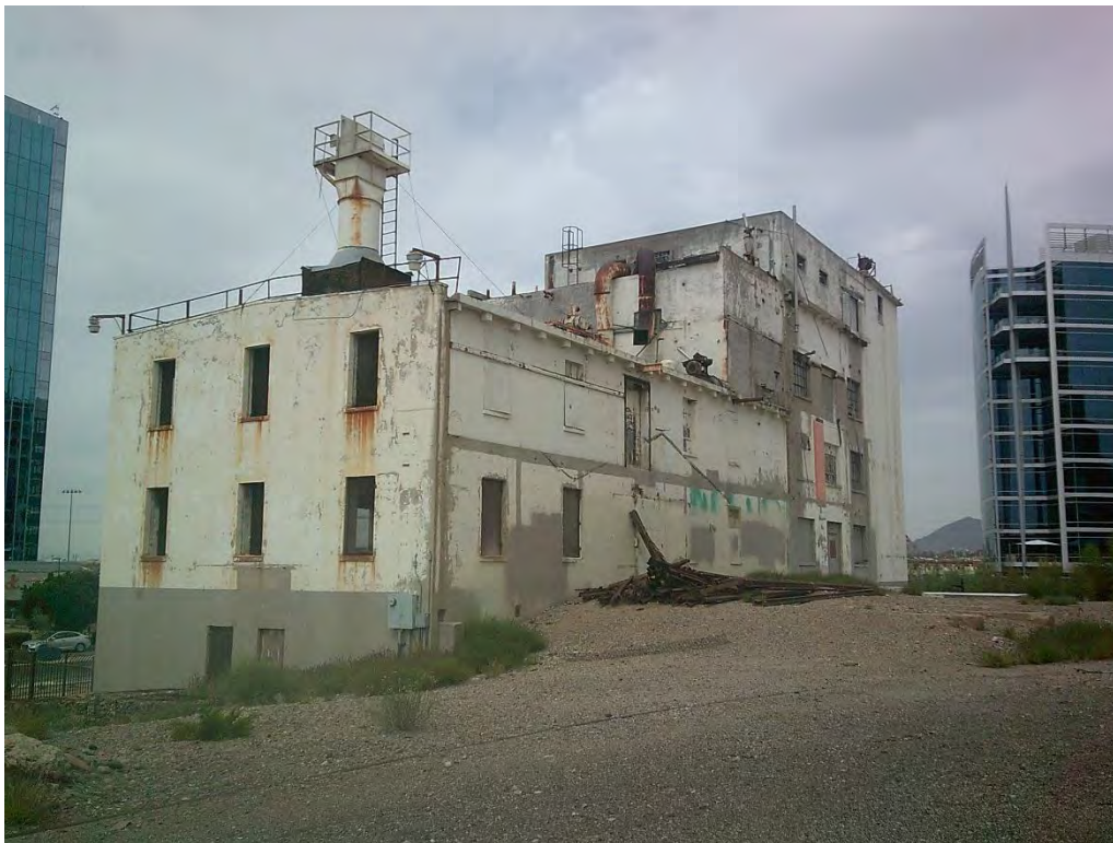
Hayden Flour Mill, 1918 building south and east elevation, view facing northwest (WestLand Engineering & Environmental Services, March 14, 2024)
