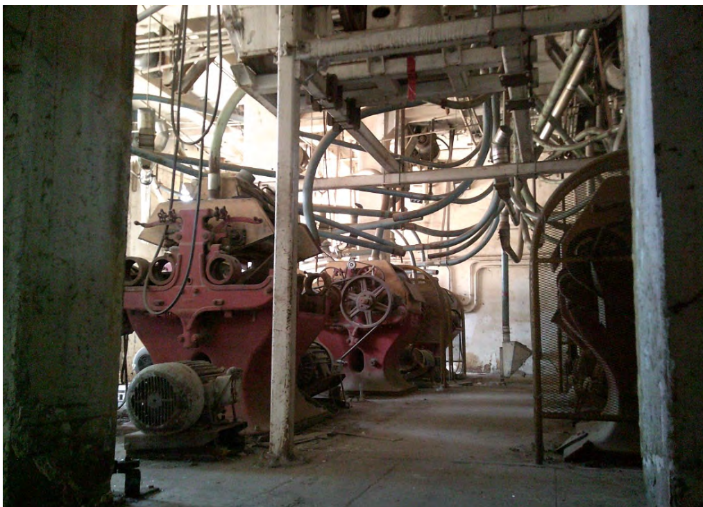
Photograph 6. Example of grinding equipment on ground floor, north half of building, view facing north (AZ_MaricopaCounty_HaydenFlourMill_006)
