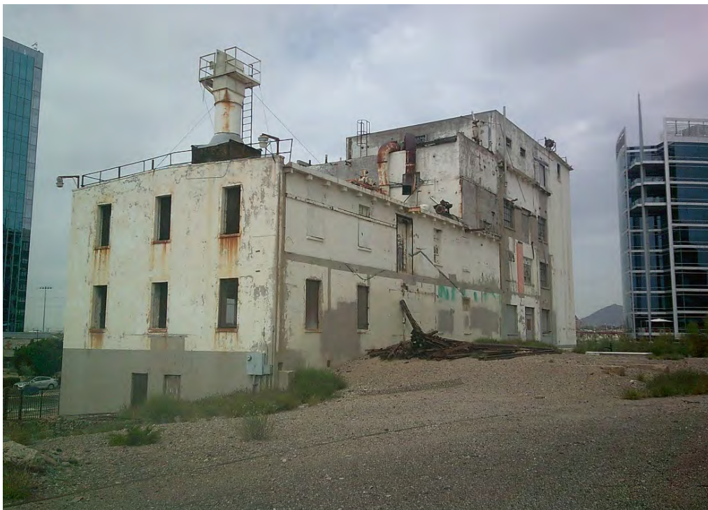
Photograph 2b. Overview of east and south elevations of mill building, view facing northwest (AZ_MaricopaCounty_HaydenFlourMill_002b)
