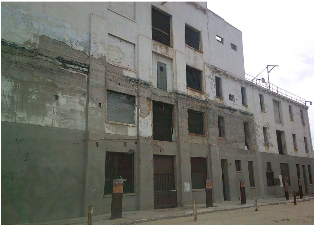
Photograph 3. Details of west elevation showing concrete pilasters and dentils along the parapet, view facing south-southeast (AZ_PimaCounty_HaydenFlourMill_003)
