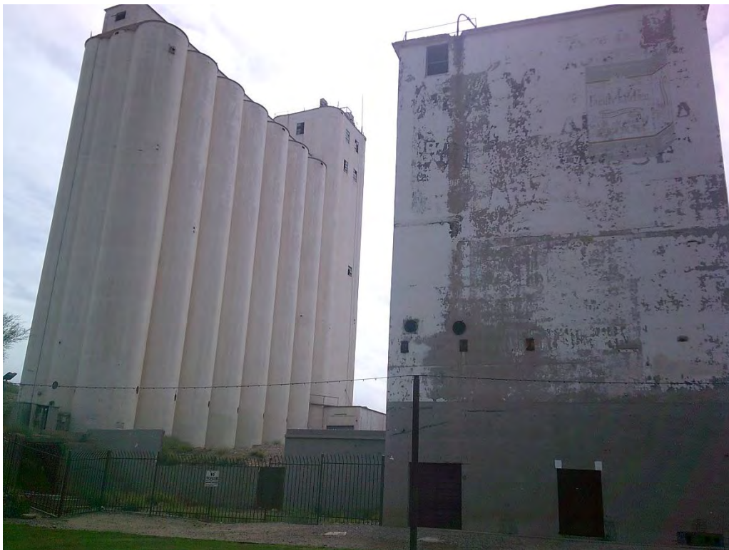
Hayden Flour Mill, overview of flour mill and silos, view facing south-southeast (WestLand Engineering & Environmental Services, March 14, 2024)
