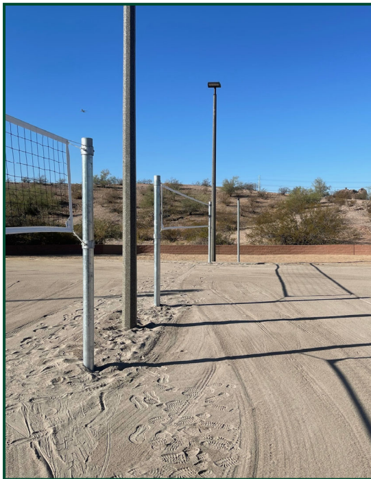
Lighting coupled with the new court wetting system at the sand volleyball courts
