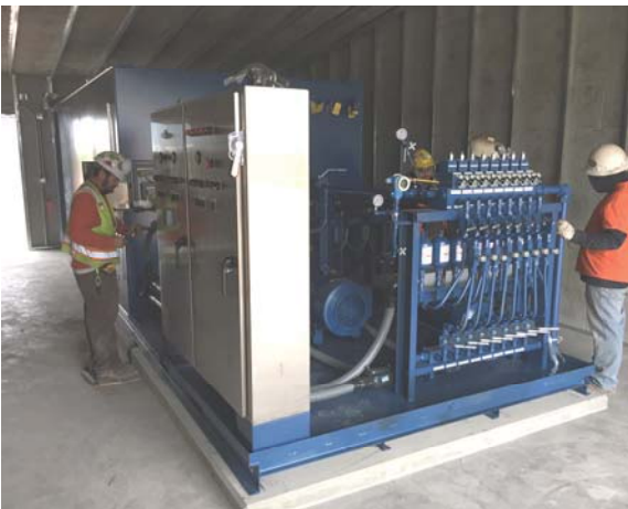
HPU (Hydraulic Power Unit) installed in the control building
