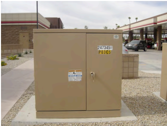
Photograph - East Transformer (1)
