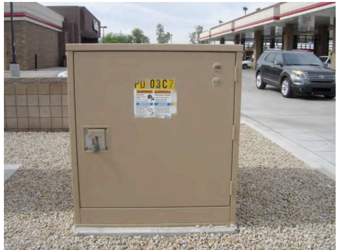
Photograph - East Transformer (2)
