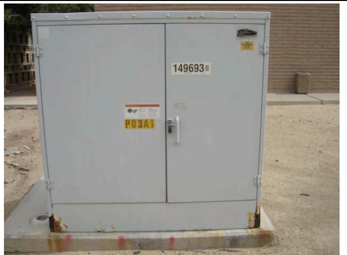
Photograph - West Transformer
