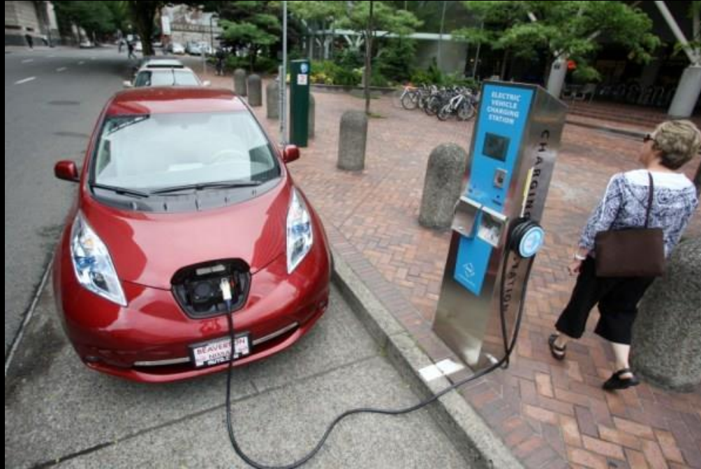
Electric Vehicle Charging Stations
