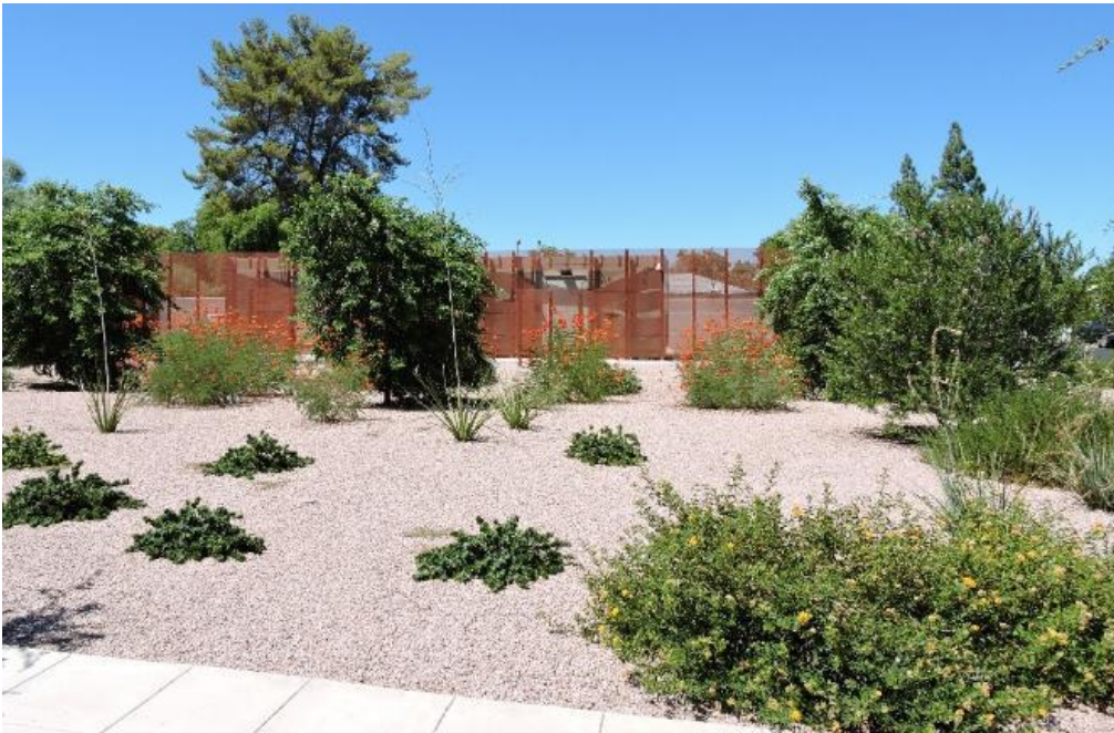
Typical TPSS surrounded by screen and landscaping
