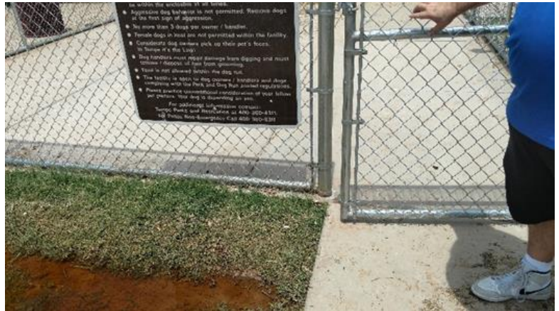
At Clark Park, the gate to the dog park is missing the required 18" clear space on the pull side of the gate.
