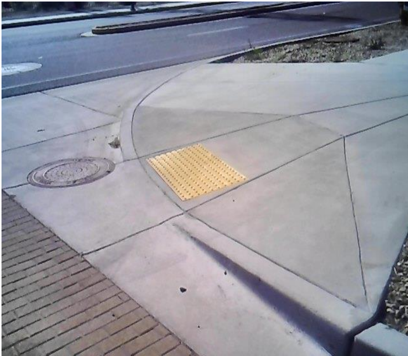
Compliant Perpendicular Ramp
