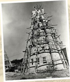
The Wigwam Lodge under construction in 1946. During this time Apache Boulevard was part of Interstate Highway 60, 70, and 80. Several of these teepee-shaped motels were built along the nation's highway system.
