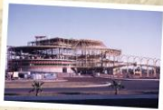
Construction of Grady Gammage Memorial Auditorium began in 1962 and took 25 months to complete.
