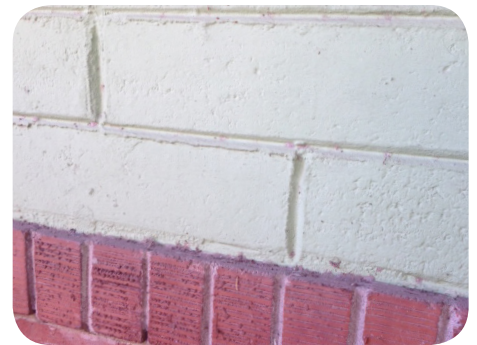
Historic building materials for the Tomlinson Estates neighborhood include masonry brick and painted concrete block.
