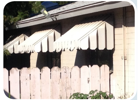
A vital detail of the historic ranch home are the awnings that shade the historic steel casement windows.
