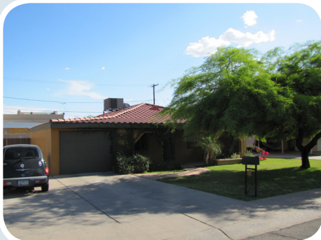
Shown above is a property that replaced its original asphalt shingles with tile ones. This alteration is not compliant with the design guidelines set forth by the community.
