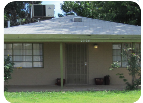
The front door on this home is covered by a screen door. These doors must be unobtrusive enough that one can still see the front door detail from the street through the closed screen door.
