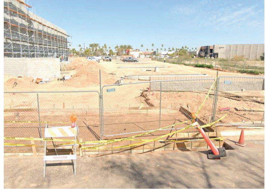
Photo 6: Facing North overlooking the Eos/Residence Inn shared driveway entrance at the South side of property.
