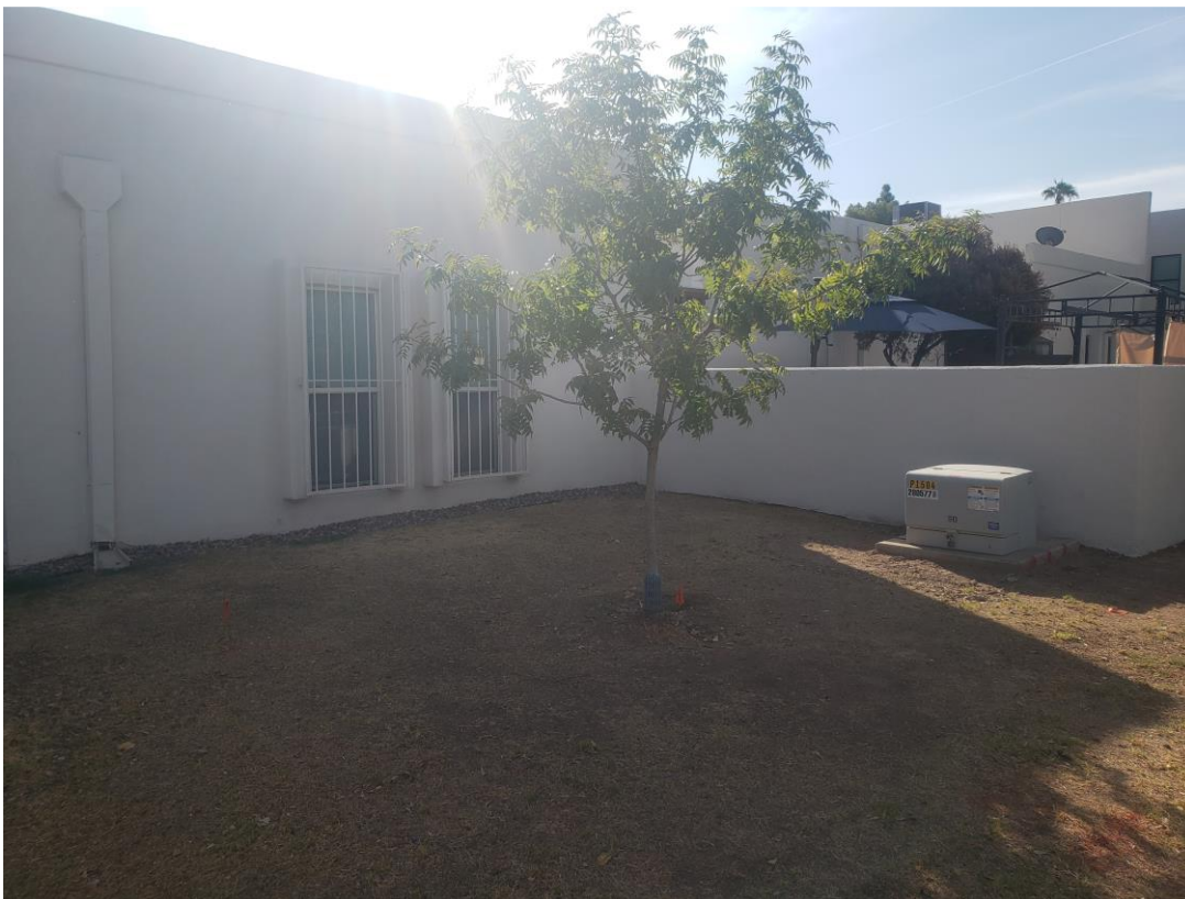
Picture 3 of 4: From the northwest corner of the property, facing southeast. The extended wall will go behind (to the east of) the SRP transformer and tree pictured to provide SRP sufficient clearance to access the transformer, then turn east so that it is in line with the east side of the current wall before joining the wall to the north.
