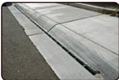
Rolled Curb & Stormwater
