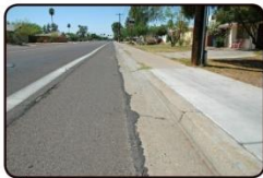
Rolled Curbing Anomaly
