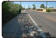
Curb Cut with No Access
