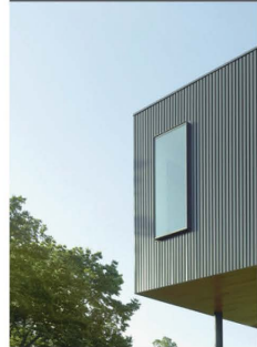
WDW-1: BLACK ANODIZED ALUMINUM WINDOW FRAME W/ 1" INSULATED GLASS W/ LOW-E COATING
