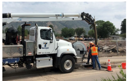
Tempe Municipal Utilities employees Robert Rascon and Raul Luna vacuum and clean a storm drain line in Flagstaff, Arizona.
