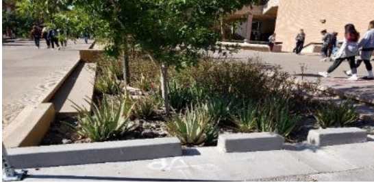
Rainwater redirect to landscaping
