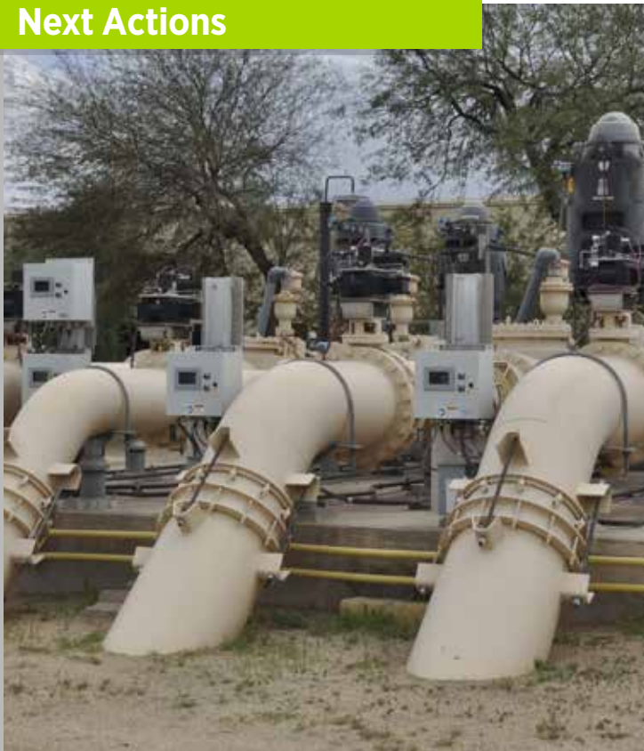
Municipal Utilities water pumps
