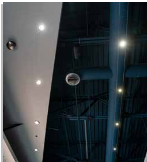
Energy efficient lighting at a Tempe small business.
