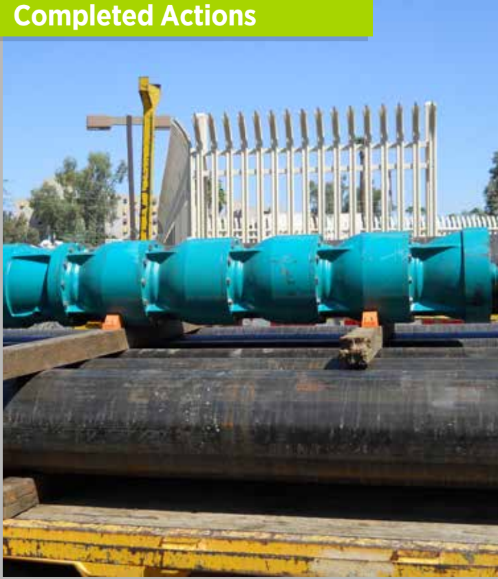
Municipal Utilities water well
