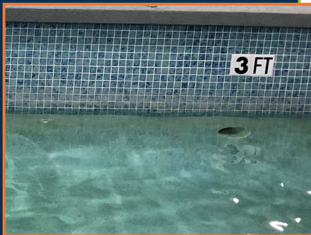
Fading and Chipping Tile
