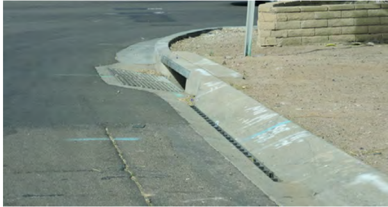
Figure 2. Typical Combination Inlet with Slotted Drain found at 3 rd Street and McClintock
