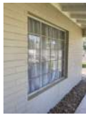
WINDOWS ALL EXISTING WINDOWS ARE STEEL PICTURE WINDOWS AND CASEMENT WINDOWS SCHEDULED TO REMAIN AND TO BE PAINTED TO MATCH THE BUILDING FASCIA.
