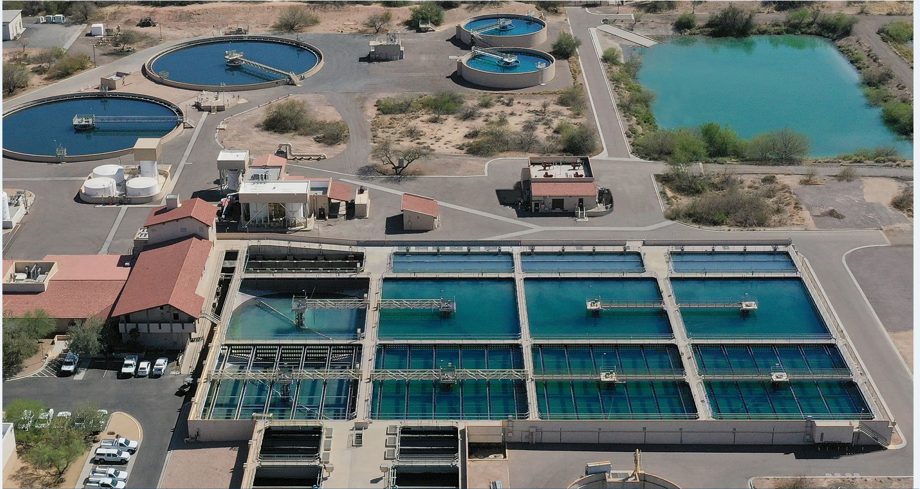
South Tempe Water Treatment Plant treats water to highest quality standards.
