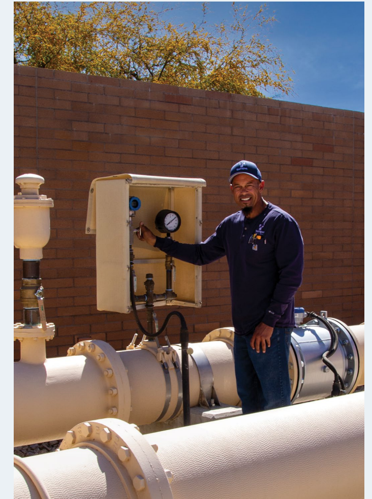
Instrumentation and Control Technician inspects meter at well site.
