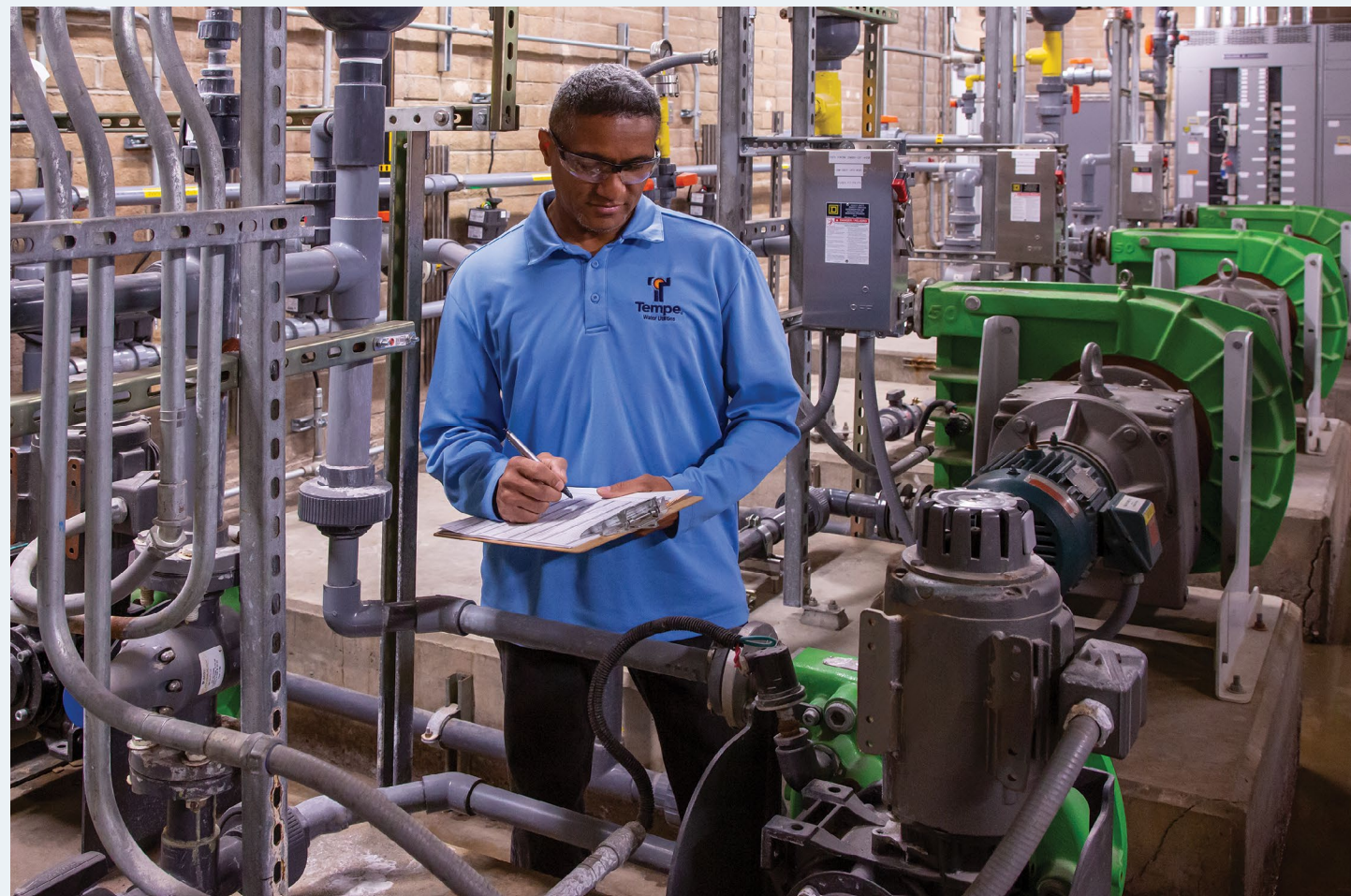
Plant Operator checks disinfection equipment.
