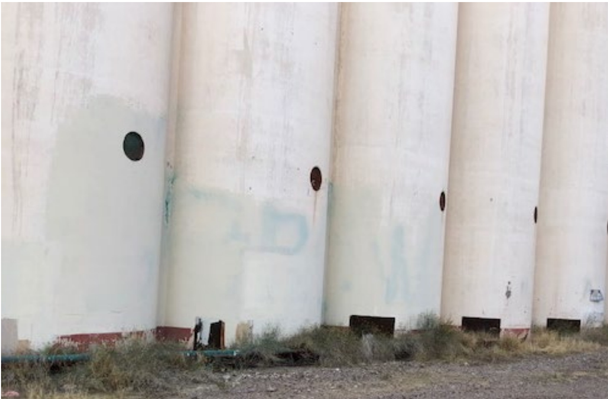
Figure 4. Photograph of exterior graffiti on the west elevation of the silos (Area 3) that had been previously painted over as an abatement strategy. Photograph taken on April 16, 2021, facing southeast.
