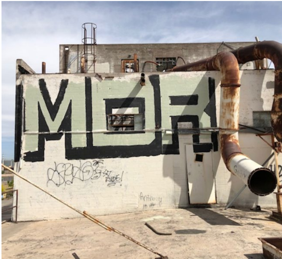
Figure 3. Photograph of exterior graffiti on the south-facing roof area the mill complex (Area 2). Photograph taken on April 16, 2021, facing north.
