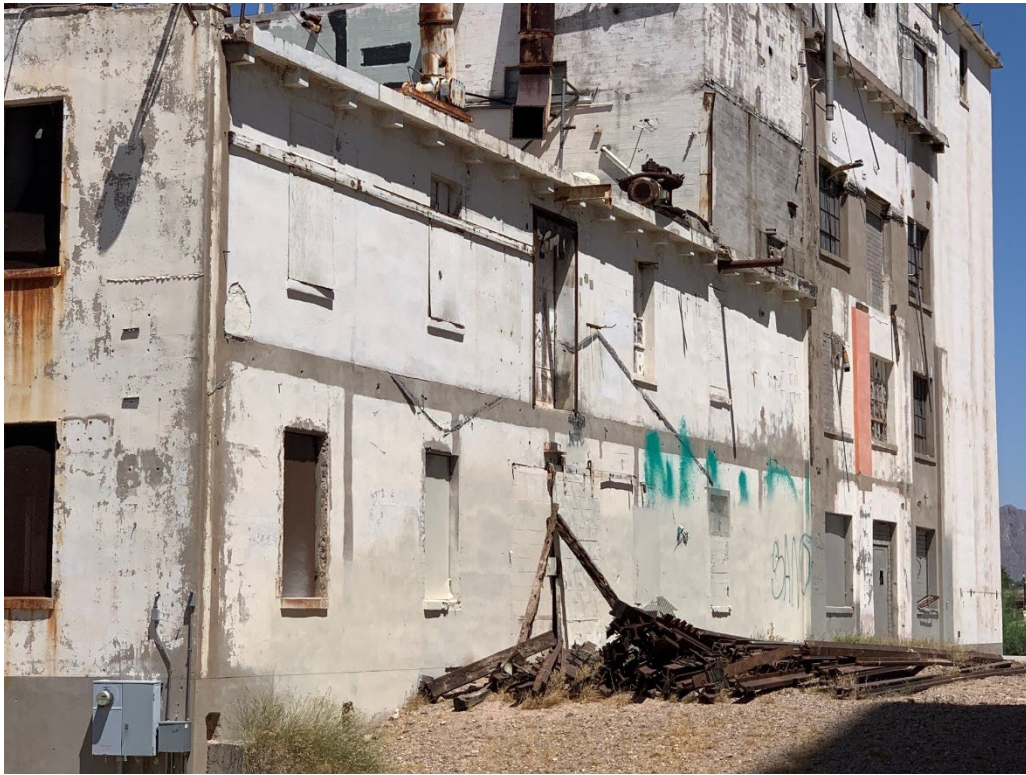
Figure 5. Photograph showing exterior graffiti tags on the east elevation of the mill complex (Area 1), including the area where the city's earlier painting-over effort is incomplete. Photograph on June 13, 2022, facing northwest.
