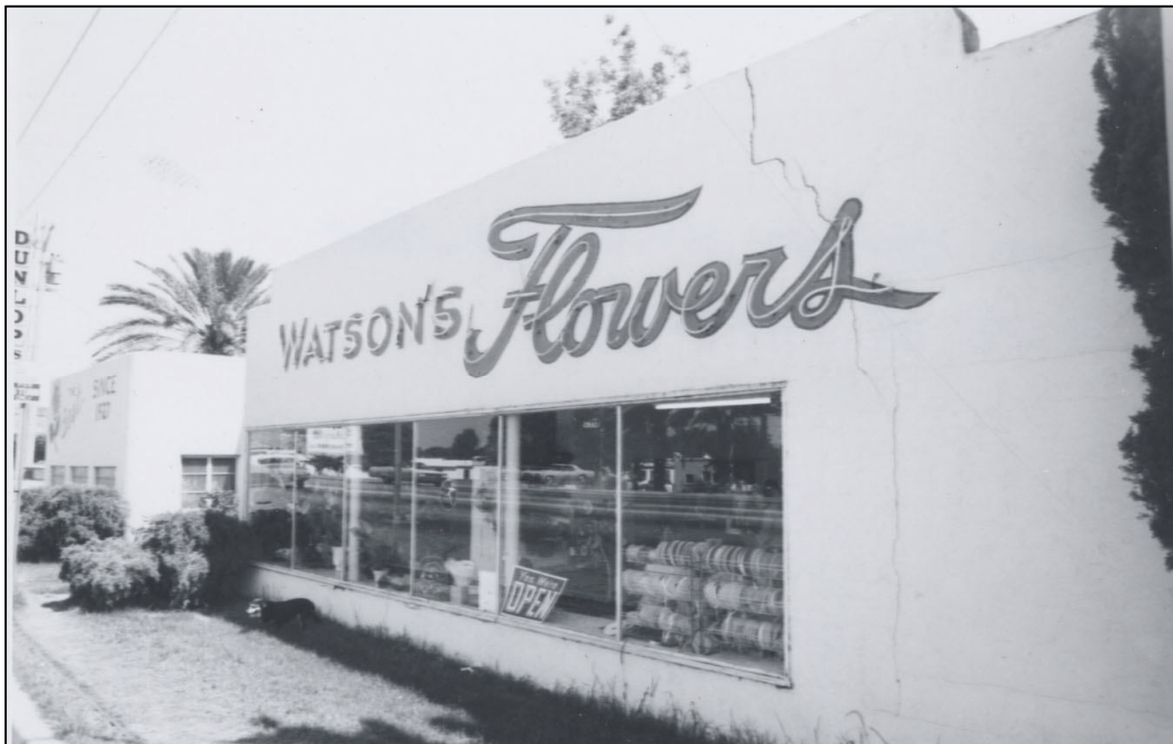
Figure 3. 1973 photograph of the western (volume) portion of Watson's Flowers, view facing southeast.
