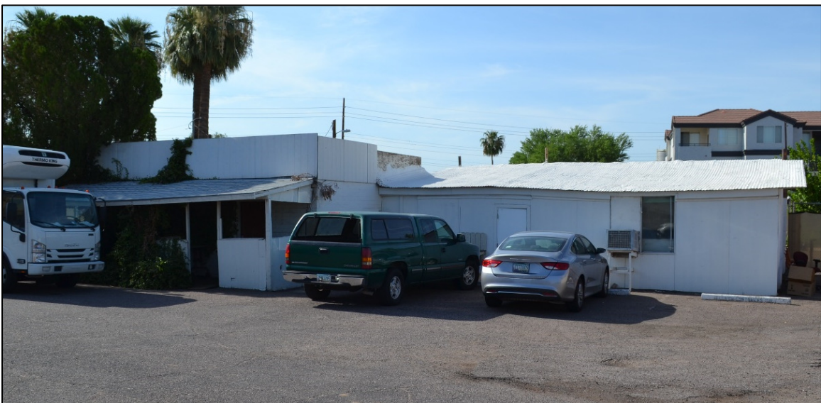
Figure 12. Overview of Building 1c, featuring a wood-framed west addition with a side gable roof (corrugated metal sheathing). View facing southeast.
