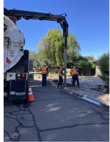
With so much complexity and so many pipes working to serve our community, water main breaks can happen anywhere and at any time.
